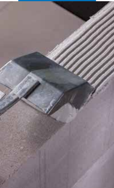
Laying Porocol FF on the surface of the wall with a special notched trowel
